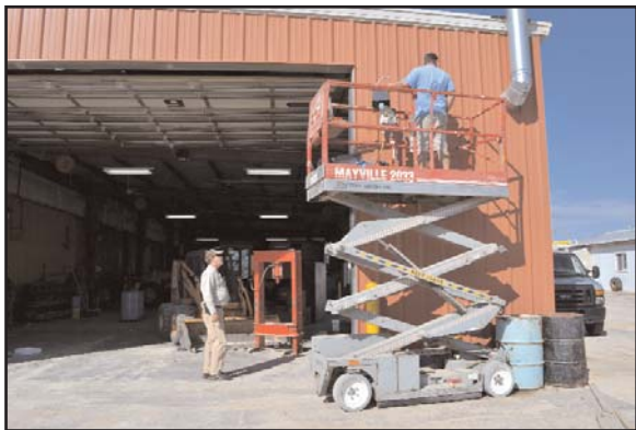
(Above) Jim Harvey (left) and Shawn Kelly (right) placing security lights on the south side of the Road & Bridge headquarters building. Harvey works for the PBPB and Kelly owns Kelly Electric in Topeka.
